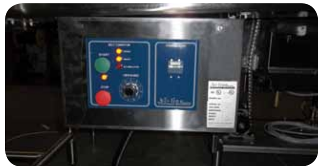
Control panel with variable speed control
